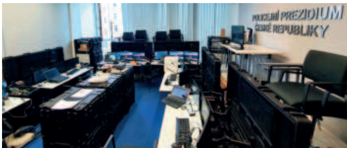
Three transportable sets (two work positions each) configured as an integrated operations center substitute in case of emergency.
