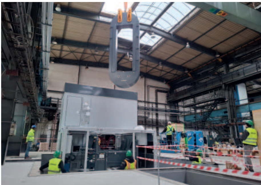
PBS Velka Bites – installation of the Quintus HIP furnace in the new hall DLT2 II.
