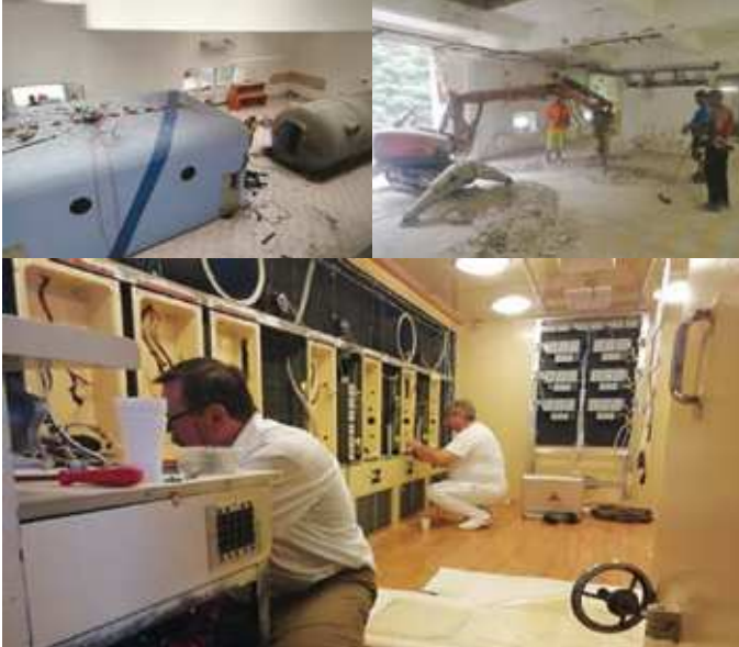
The original chambers were disassembled part by part because of the conservation of some elements and also because of potential hazardous materials.
